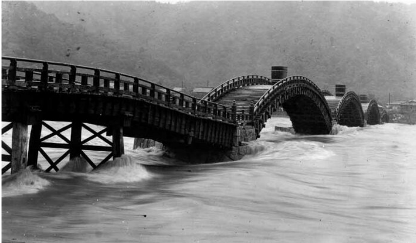
Figure 15 Loss of one pier before collapse (1950)
