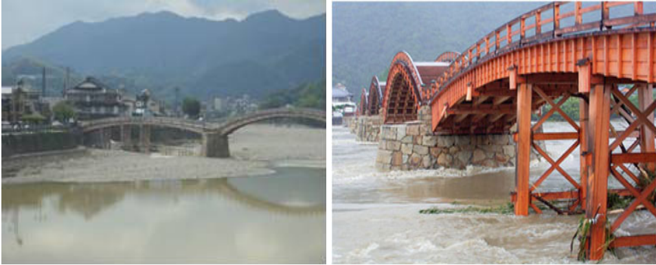
Figure 16 Loss of two piers reducing damages (2005) (see online version for colours)
