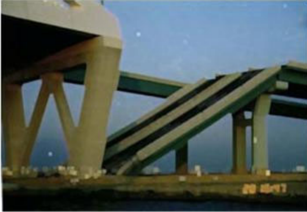
Figure 2 The Hyogo-ken Nanbu earthquake (1995) (see online version for colours)
