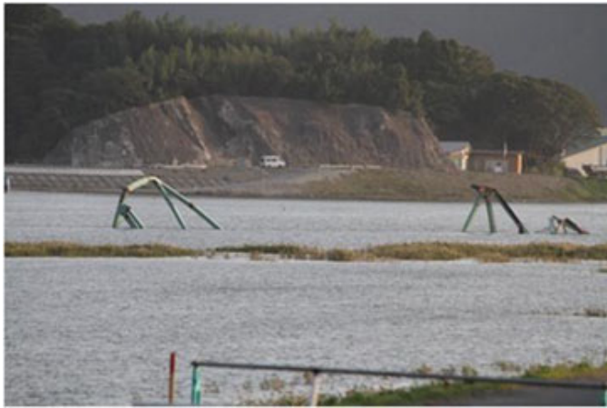
Figure 13 Truss members being swept away (see online version for colours)
