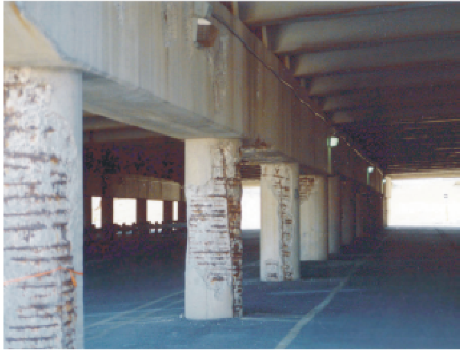
Figure 1 Highway bridge columns deteriorated as a result of steel corrosion (see online version for colours)
