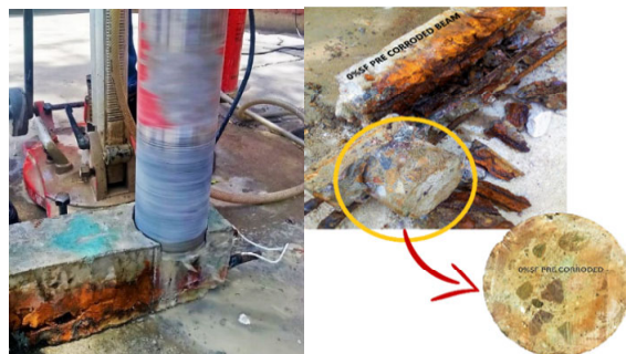
Figure 5 Core extraction from the tested RC beams for pre-corroded and loaded specimens (see online version for colours)
