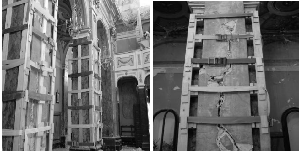
Figure 7 Observed damages after the 2009 seismic event on rubble masonry pillars of St. Gemma (SGM) church in Goriano Sicoli (AQ)
