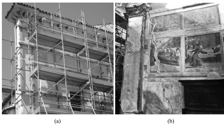
Figure 9 (a) Top-corner overturning on St. Maria della Pace church in Capestrano and (b) apse overturning on SMA church in Gagliano Aterno
