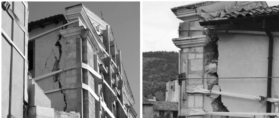
Figure 8 Façade overturning in SGM church in Goriano Sicoli (AQ)
