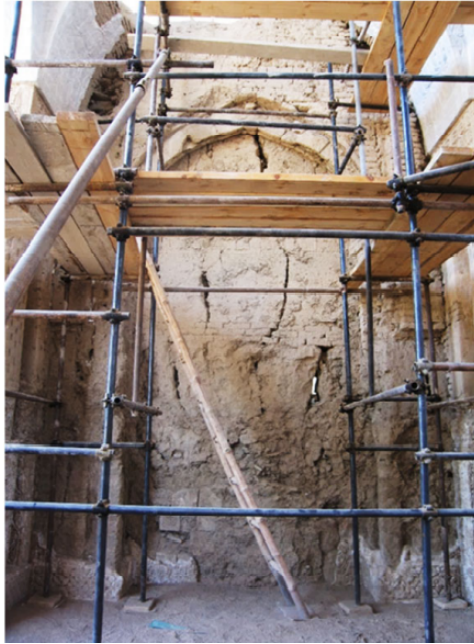
Figure 6 Conservation state of the wall constituting a niche (see online version for colours)
